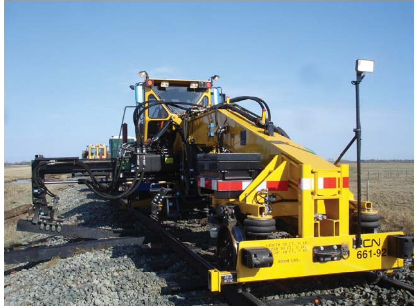
TRIPP - Tie Exchanger
