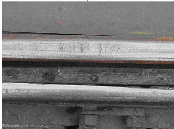
Thermal cracks on burned stock rail
