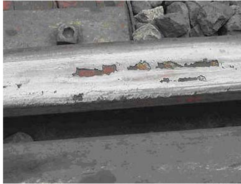
Flattened rail head showing displacement of parent metal (spalling)
