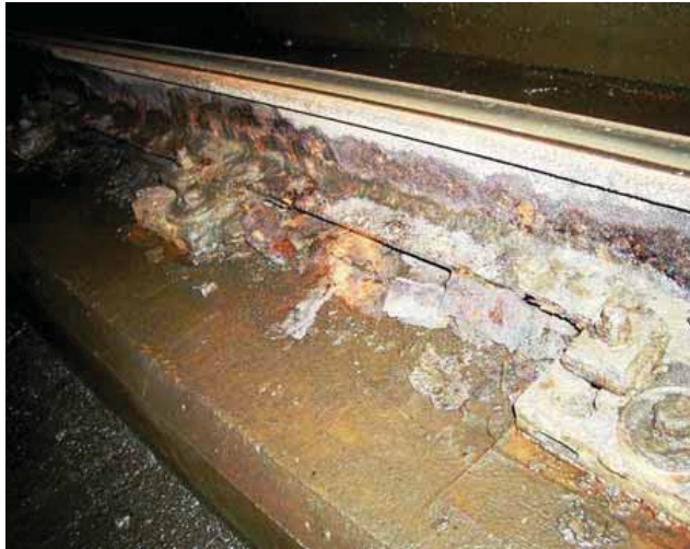
Corrosion on rail, fastening systems, and plates
