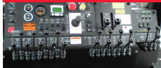
Rebuilt Ballast Regulator operator panel
